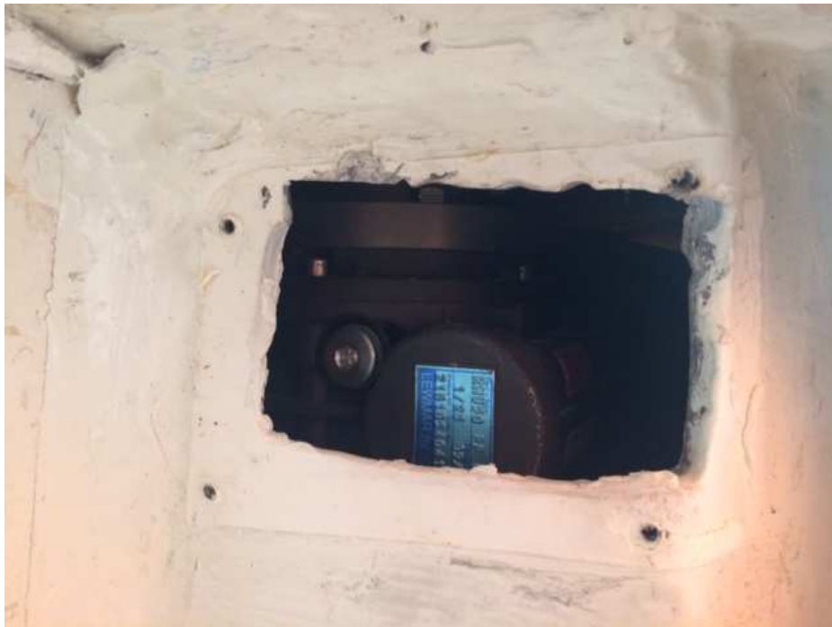
Inspection hatch for access to the motor
