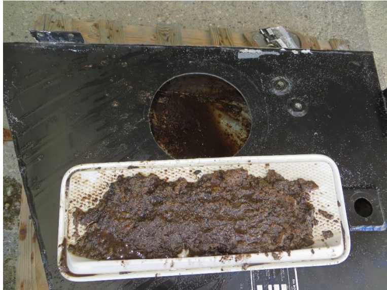
Slimy substance on tank wall and bottom due to micro-organisms
