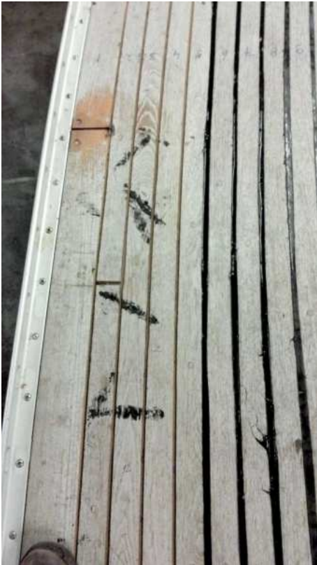
Fig. 17 'Stepped in the caulk' and left traces
